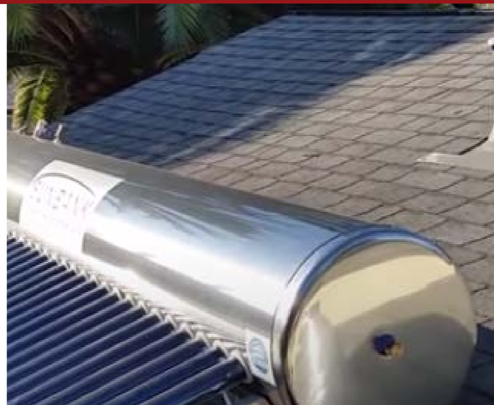
Water heating solar system
